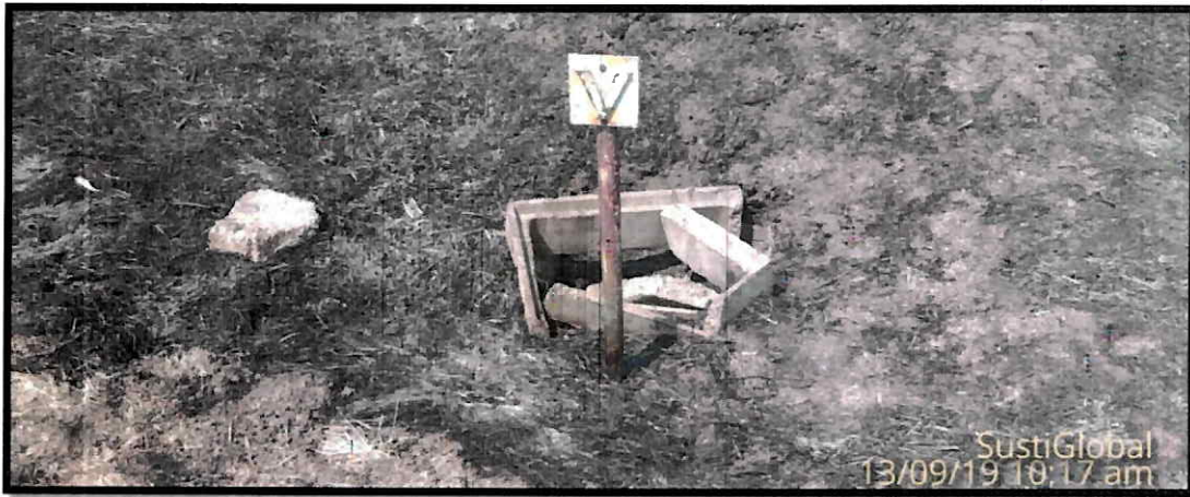
Plate 3.1: Nearby portable water valve (photo by consultant)
